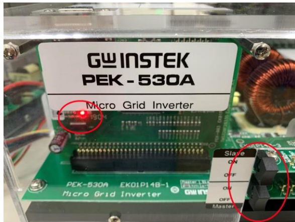
Figure 4.7 DSP normal status with light on
